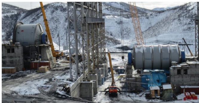
Semi-turnkey gold ore grinding plant with a production capacity of 1.300 tph, semi-autogenous mill with 15 MW and ball mill with 18 MW / Russia
