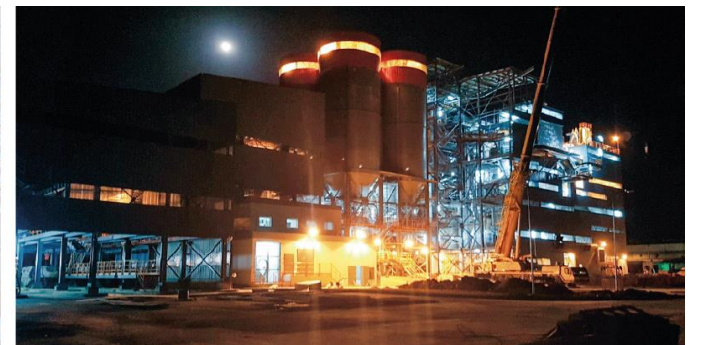
Turnkey cement grinding plant with a production capacity of 135 tph, ball mill (inside Ø: 4.6 m, length: 15 m, drive power: 4.700 KW) / Ghana
