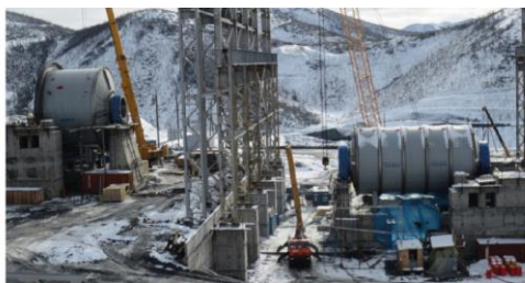
Semi-turnkey gold ore grinding plant with a production capacity of 1.300 tph, semi-autogenous mill with 15 MW and ball mill with 18 MW / Russia
